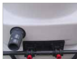
WATER FLOW VALVE
