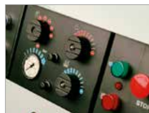
CONTROL PANEL PROVIDED WITH EMERGENCY SHUTDOWN
